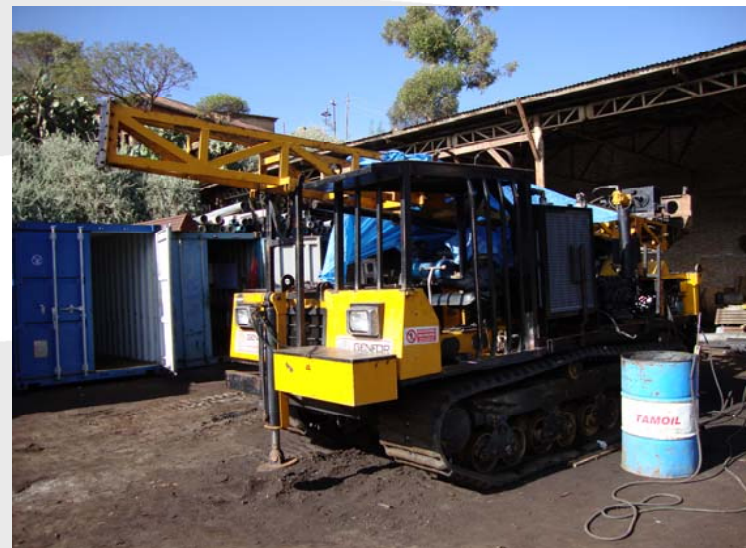
General Exploration Drilling – diamond drill rig for the Colluli Potash Project, Eritrea.
