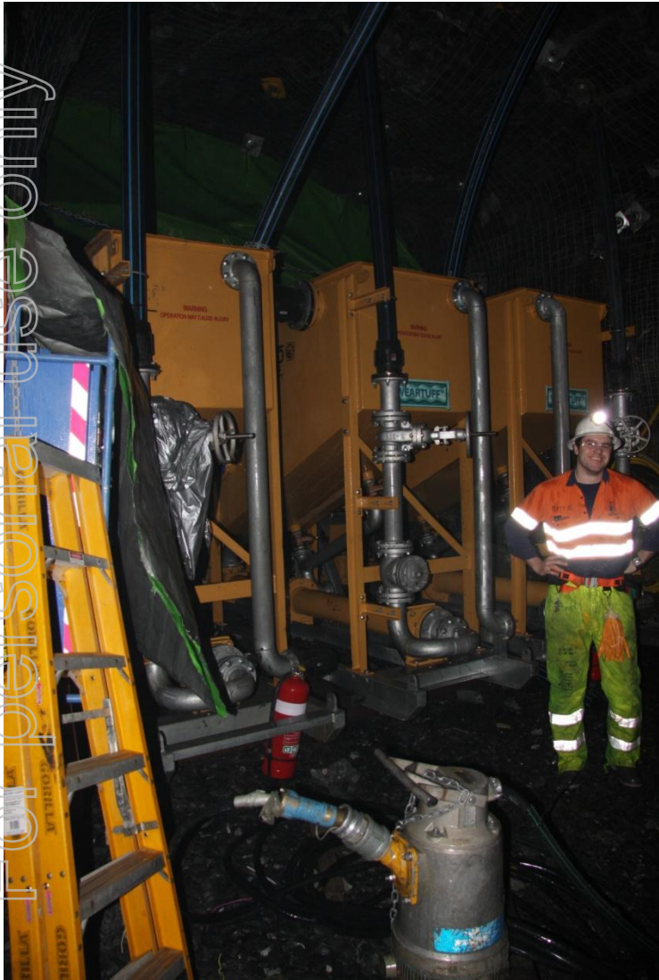
Underground water pumping station www.bassmetals.com.au
