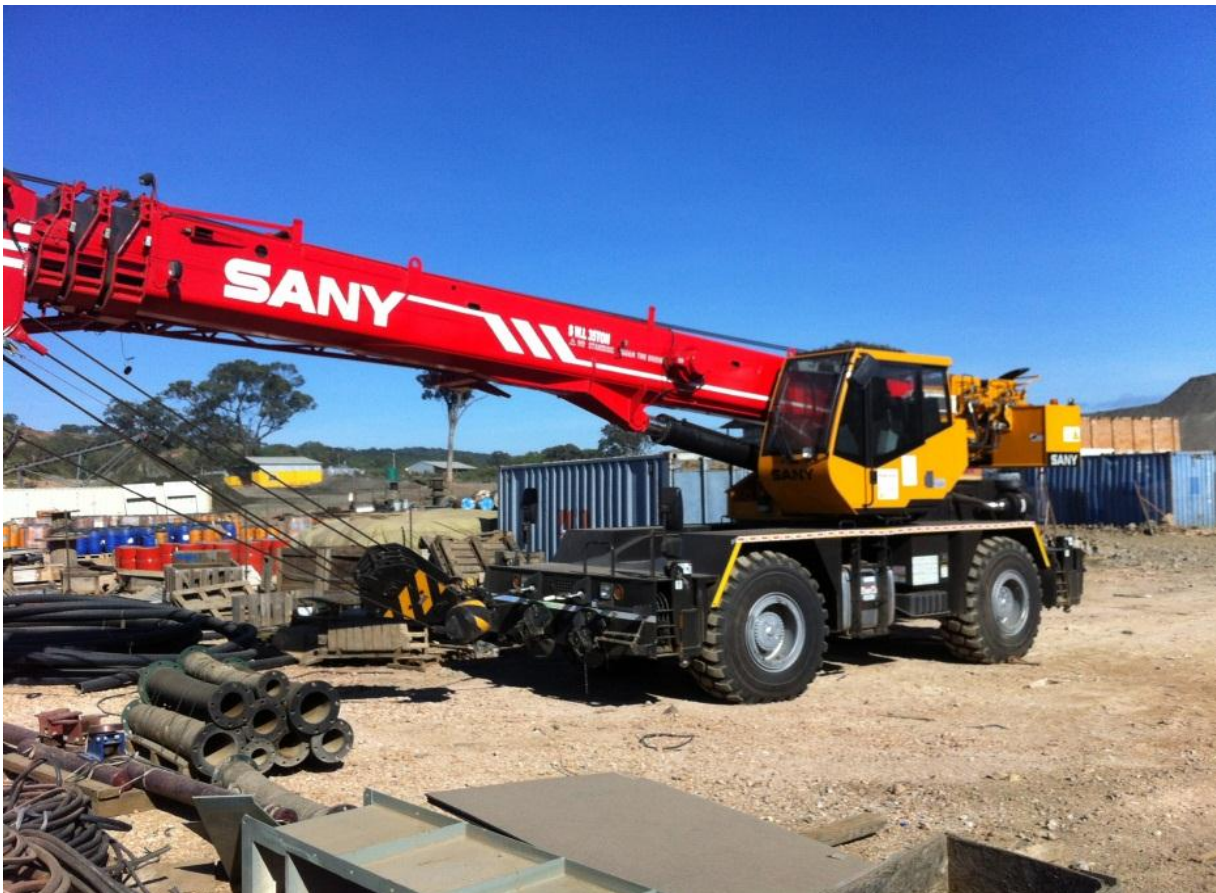
The 35t crane for the erection of the SXEW plant at the Kipoi bonded customs clearing facility
