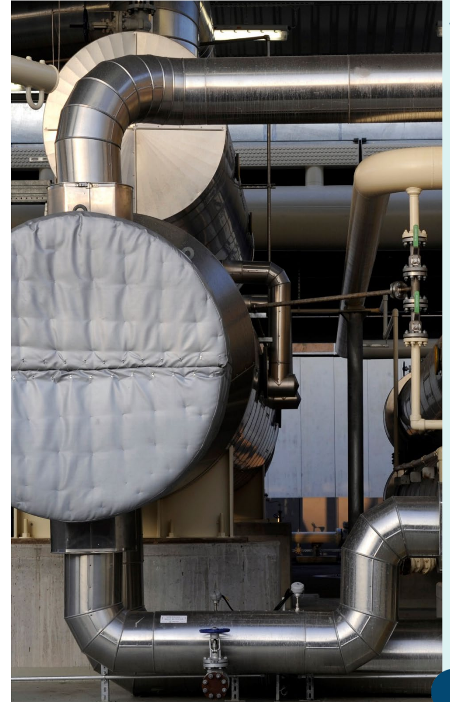
Vulcan's Insheim Geothermal Power Plant
